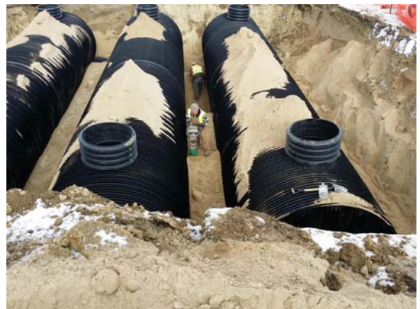
Underground tanks at Bayview Elementary School collect stormwater for irrigation reuse.
